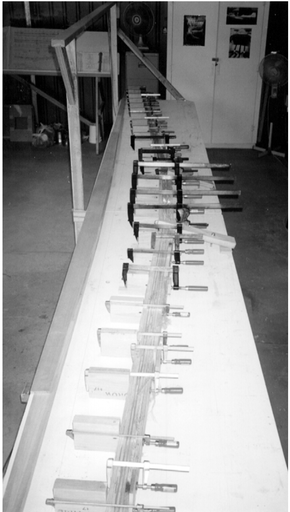
Neil Aitkenhead's main wing spar laminations being glued on the jig table.
