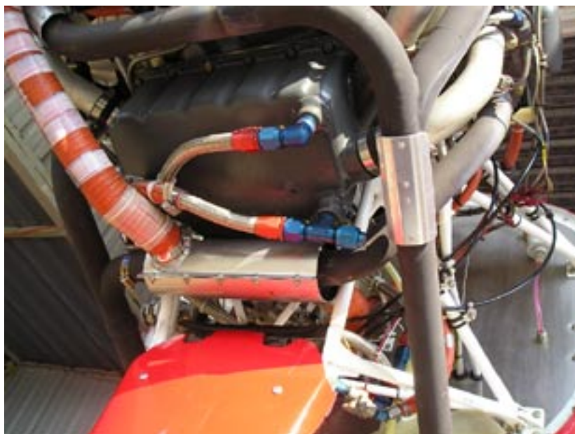
Figure 1. This shows the installation of the sump fittings on an IO-360-B1E (Dan Dorr photo)
